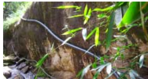
Penstock in Nedumkandam
