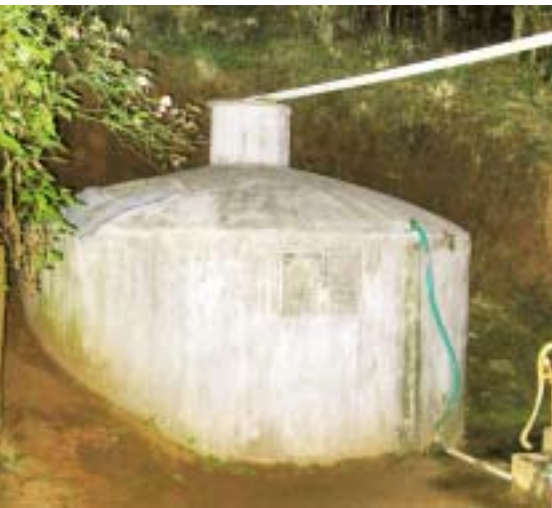
Biogas Plant initiated by MALANADU
