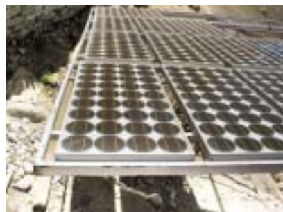
Photovoltaic cells at SECMOL, Leh
