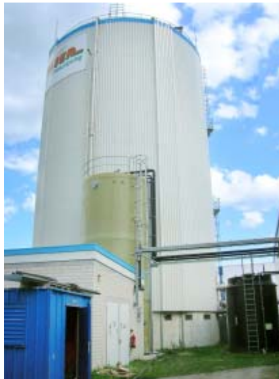
Biogas digester and engine room at BKF, Freiburg
