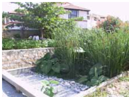
The DEWATS horizontal gravel filter can be aesthetically incorporated in the local surroundings.
